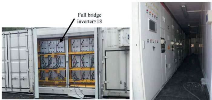
Figure 11. Appearance and internal arrangement of the DVR.
